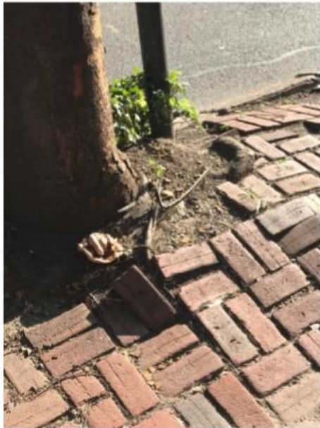
An unsafe sidewalk. San Francisco and some other cities pay to repair damage caused by tree roots. (Elise Vider photo)
