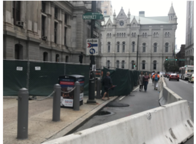
Even where sidewalks are wide and streets are wider, like at City Hall, we block them for construction. (Elise Vider photo)
