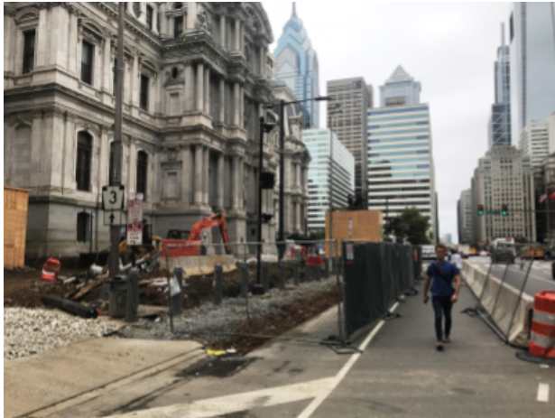
Current construction around the northeast quadrant of City Hall pushes pedestrians into the street, in a "protected" walkway. (Elise Vider photo)
